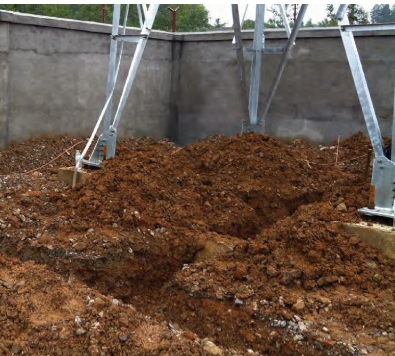
Telecom tower grounding
