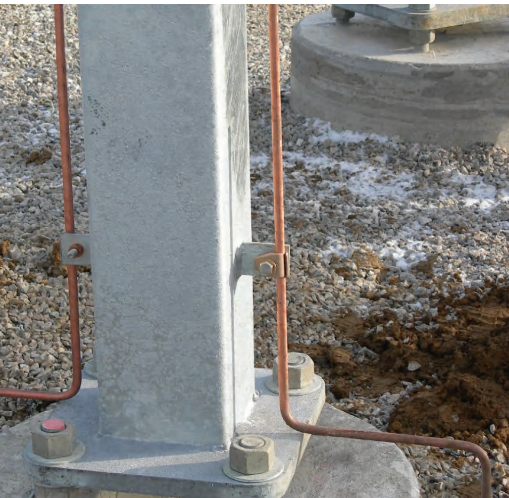
Substation earthing riser
